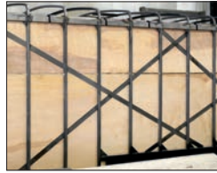
Cross Bracing Wall Gussets
